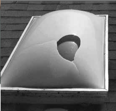
Old acrylic domes can be easily damaged.
